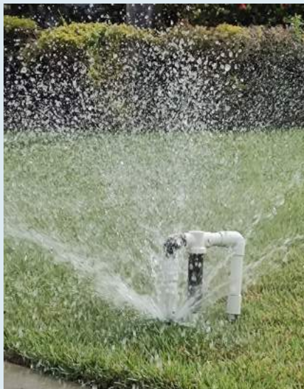
A pipe constantly under pressure burst, draining thousands of gallons before being shut off.
